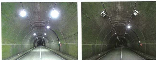
When there is a travelling vehicle(s) When there is no travelling vehicle
