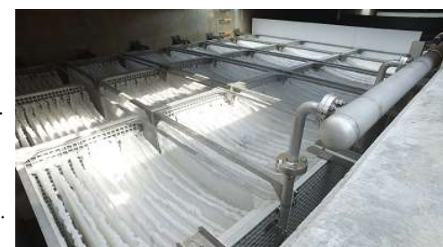
Example of installed fibrous media
