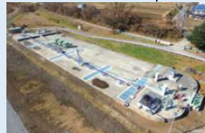
Sewage treatment facility (B-DASH project) in Japan
