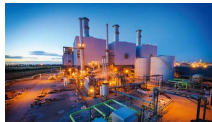
Saltend GTCC Power Plant
