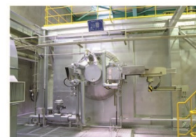
Bao hơi Boiler drum
