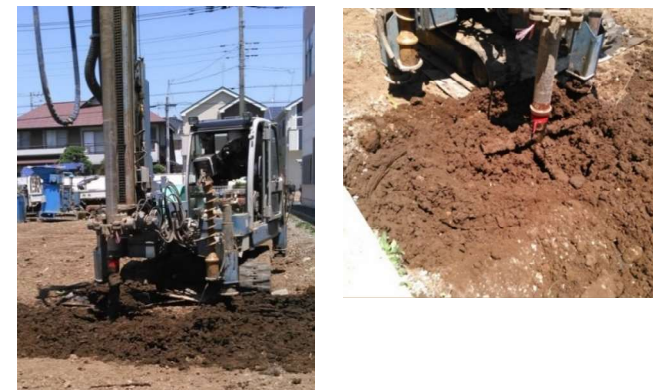
Fig. 8 Mixing of RNIP into contaminated soil with mechanical mixing or agitating method
