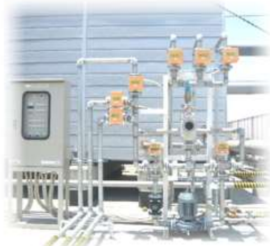
Commercial facility refrigeration
