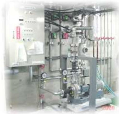
In-house underground station refrigeration
