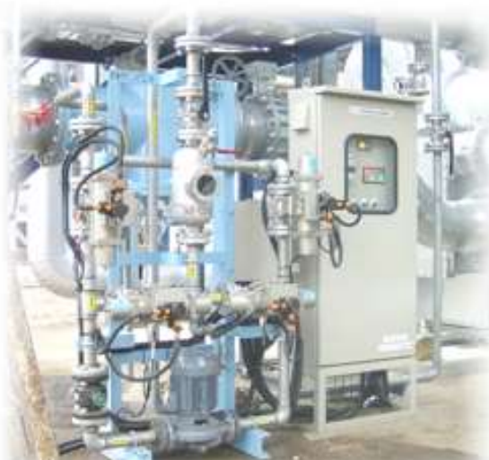
Chemical plant refrigeration
