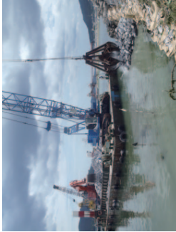
Restoring the embankment used by floating cranes at Taiheiyō Cement's Ofunato Plant
