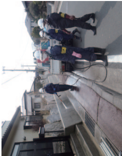
A nuclear-waste reduction experiment in a Fukushima Prefecture decontamination technology verification project
