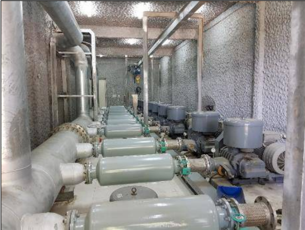
Phu Loc WWTP Air Blower ARS150 30KW x 12 units
