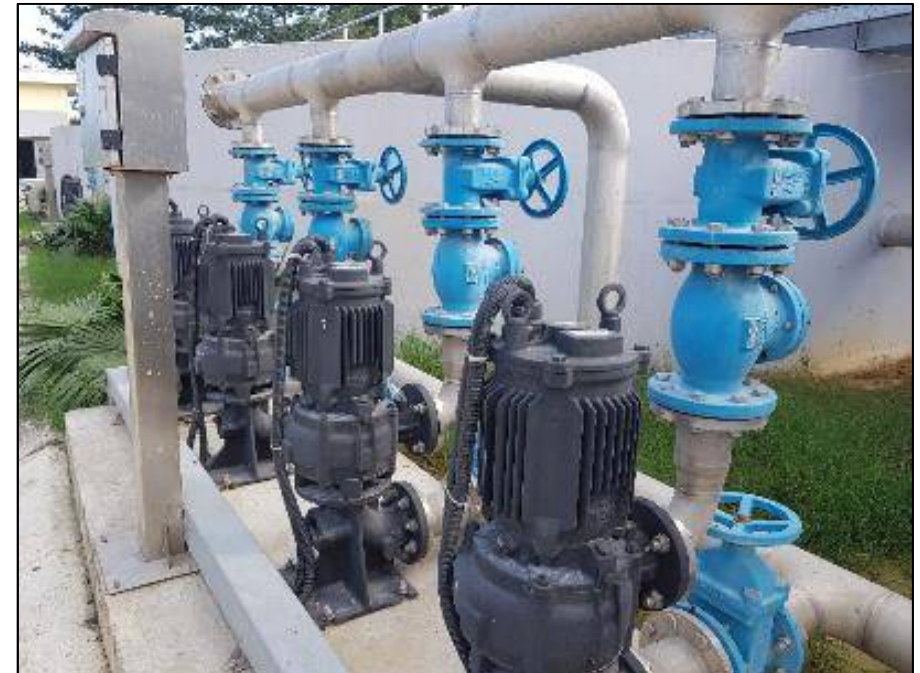
Khanh Son Garbage Treatment Plant Dry Pit type Pump x 14 units
