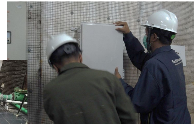
IoT monitoring system
