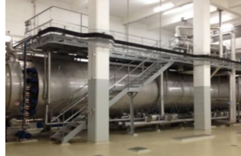
Vacuum System Improvement.
