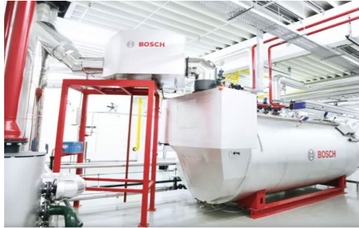
Heat Recovery flue gas
