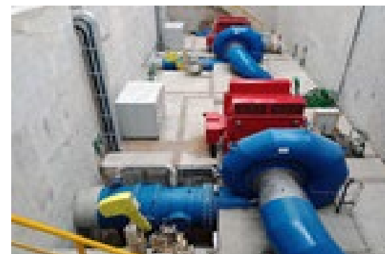
Hydro Power Plant, Toyo Energy Farm Co., Ltd., Indonesia
