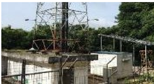
Energy-saving of mobile communications base transceiver stations, KDDI Corp. Indonesia
