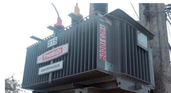
Introduction of Amorphous High Efficiency Transformers in Power Grid, Yuku Keiso Co., Ltd., ①Vietnam, ②Lao PDR
