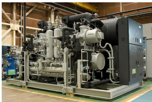
High-efficiency refrigerator, Mayekawa MFG, Indonesia
