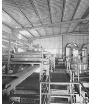
Slurry Plumbing System
