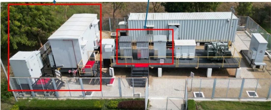
Battery banks Inverters
