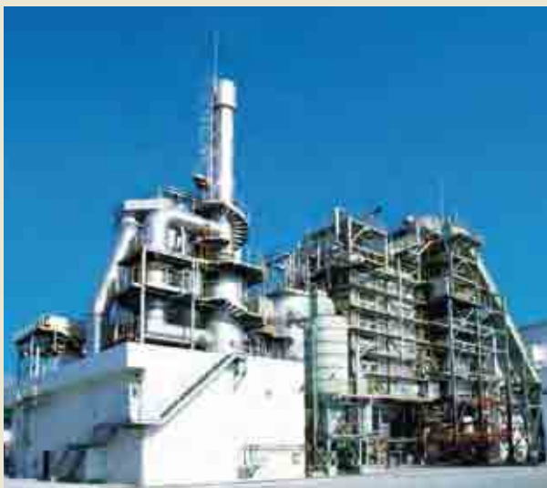
In Thailand, an industrial waste incinerator has been operating from 2006. Its treatment capacity is 100t/day. Source: JFE Engineering Corporation
