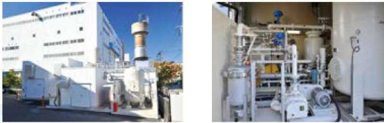
Facility for Adjustment of biogas in Japan
