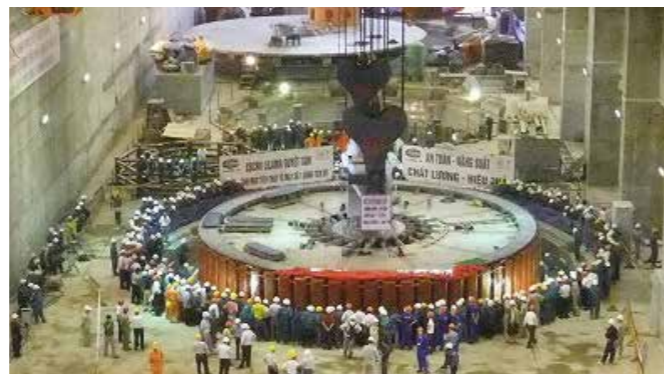
Generator in Powerhouse for Son La Hydropower Project Vietnam
