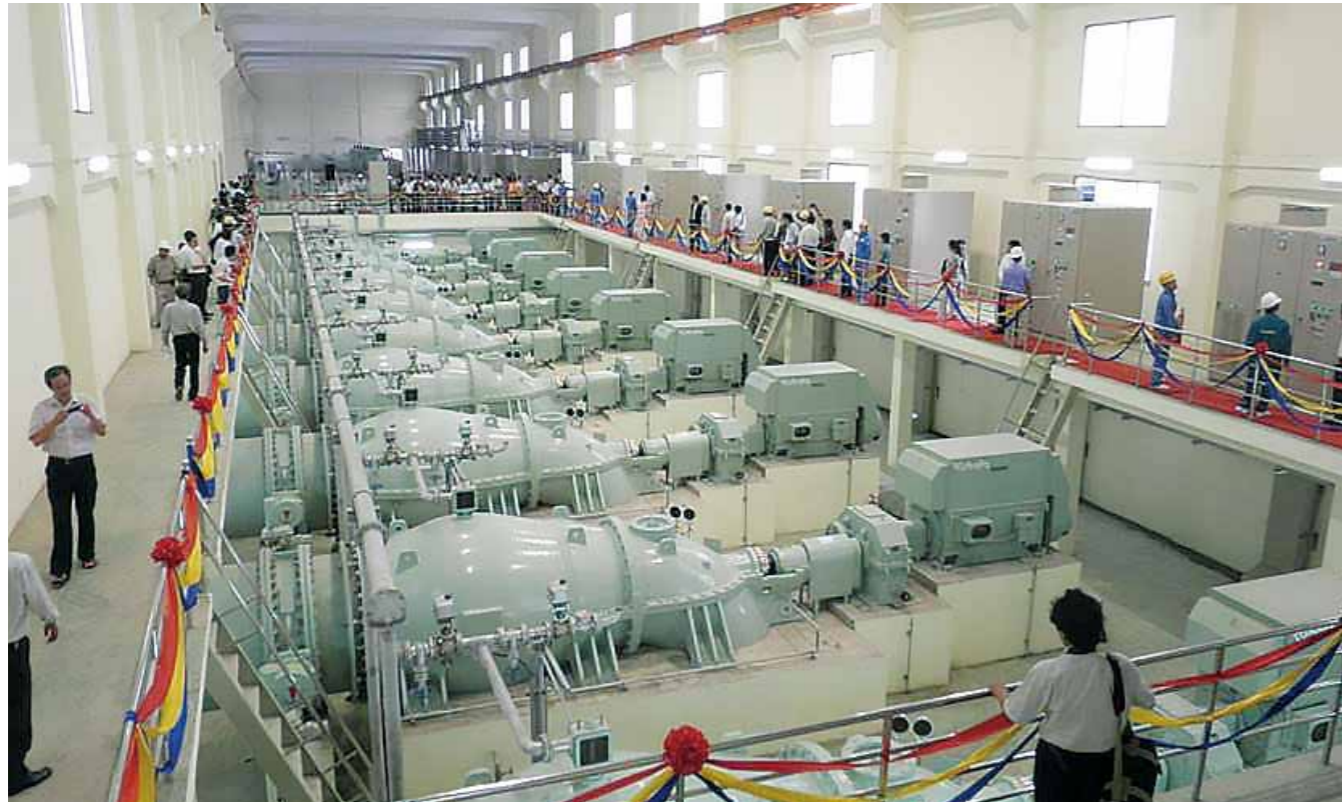
Drainage Pumping Station (90 m 3 /s), Drainage Project for Environment Improvement in Hanoi, Vietnam
