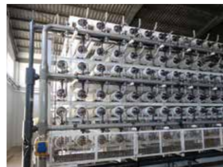
RO Unit, Water Supply System Development Project in Santiago Island, Cape Verde
