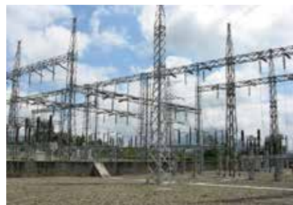
Brastage Substation, Indonesia
