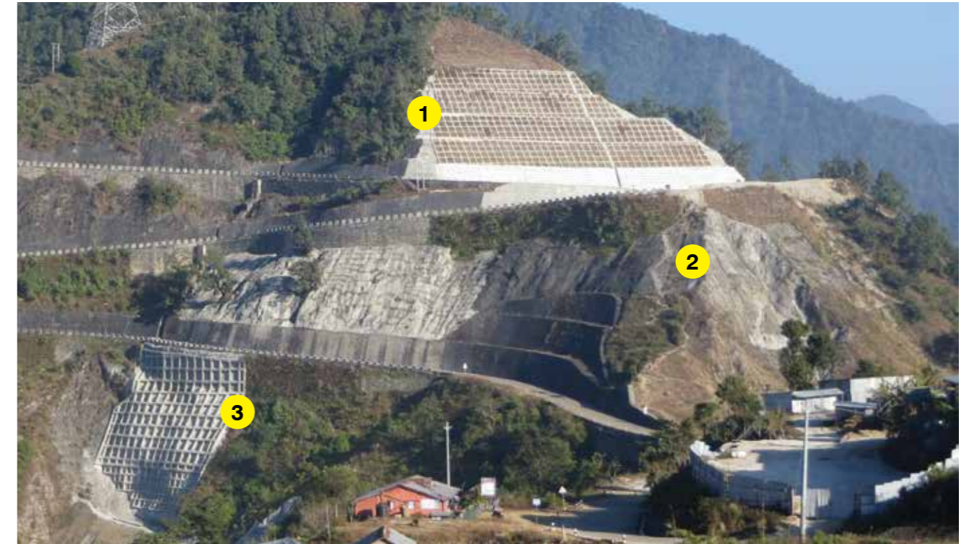
Three major Countermeasure against the Landslides and Slope Protection works . Shinduli Road Sec II, Nepal.
