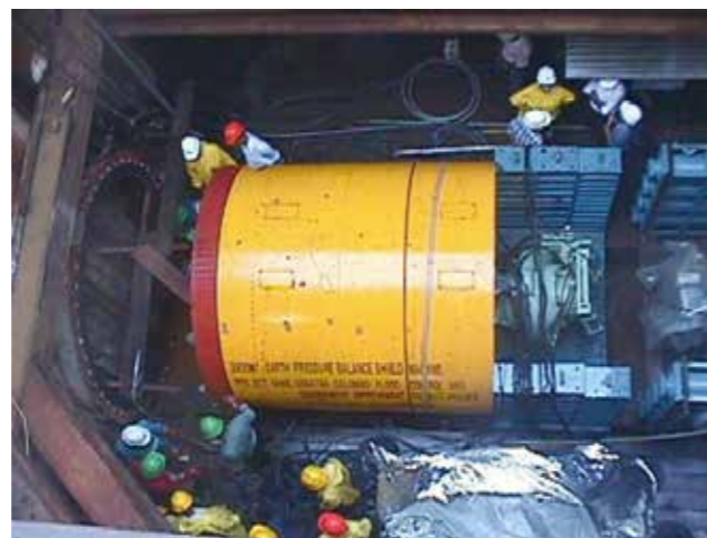
Drainage Pipe Installation, Greater Colombo Flood Control & Environmental Improvement Project, Sri Lanka
