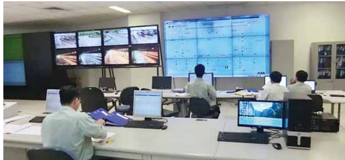
ITS equipment at Hai Van Tunnel Operation Control Center, Vietnam
