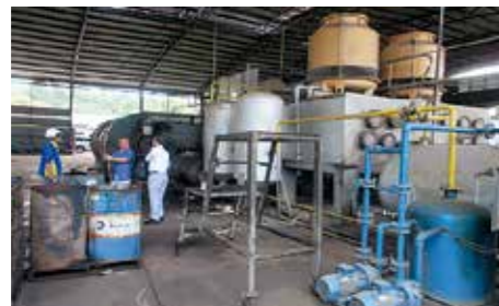
Energy reduction with high efficiency factory boiler, Indonesia
