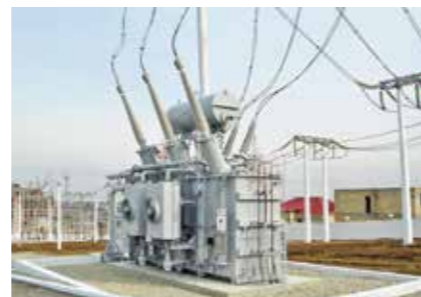
Transmission Project, Sri Lanka
