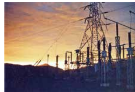
Mushviq Substation Baku, Azerbaijan
