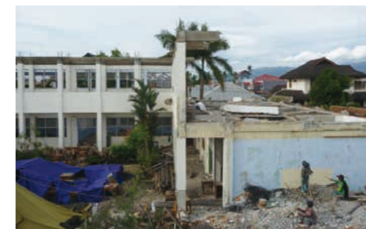
Project for the Safe School Reconstruction in Divested Areas of Earthquake in Offshore of Padang in West Sumatra Region (Indonesia)
