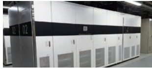
Substation Systems (UPS)
