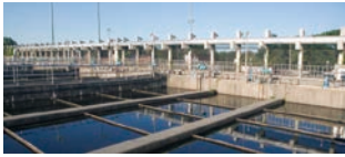
Water & Wastewater Treatment Systems
