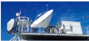
Disaster Management Systems (Radio Transmission System)
