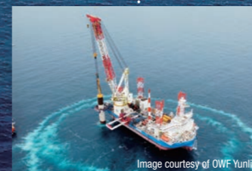
Yunlin Offshore Wind Farm Construction Project (Chartered) Greater Changhua Offshore Wind Farm Construction Project (Chartered)
