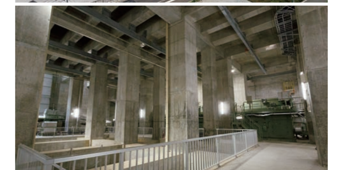
Ishinomaki Central Drainage Pump Station (Ishinomaki City, Miyagi) Exterior (top) and interior (bottom)
