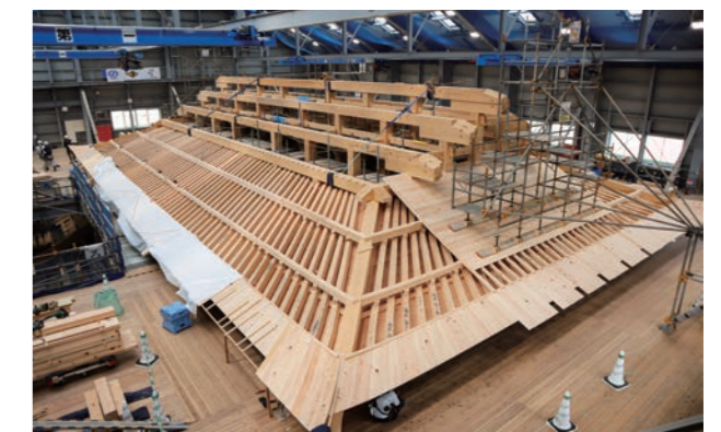
Shurijo Castle Main Hall Reconstruction Project (Naha City, Okinawa) Inside the temporary building where the construction of the wooden framework for the roof interior is progressing
