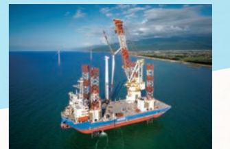
2023 Nyuzen Offshore Wind Power Farm Constructed using our self-propelled SEP vessel BLUE WIND.
