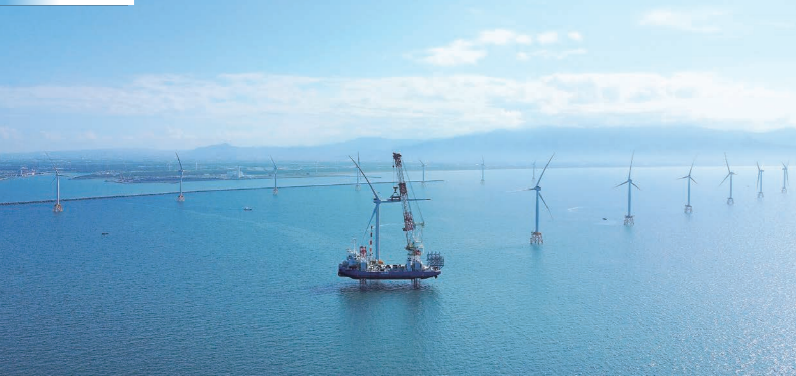
Construction of wind turbines at the Ishikari Bay New Port Offshore Wind Farm (within the Ishikari Bay New Port Harbor, Hokkaido)
