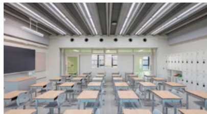
RKU Kashiwa Junior High School (HVAC and electrical work in classrooms) (Kashiwa City, Chiba)
