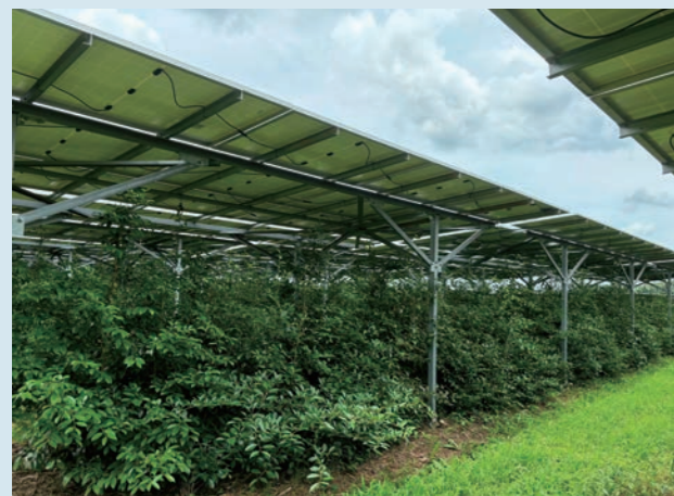
Tsukuba farm-based solar power plant (Tsukuba City, Ibaraki)
