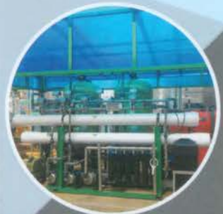
Reverse Osmosis System for Boiler Feed Water
