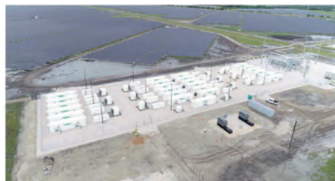
The Lily Energy Storage Project in Texas, the US
